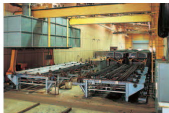
酸洗 Acid Pickling
